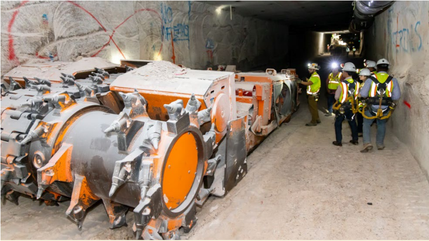
An underground continuous mining machine prepares to mine salt at the new utility shaft
