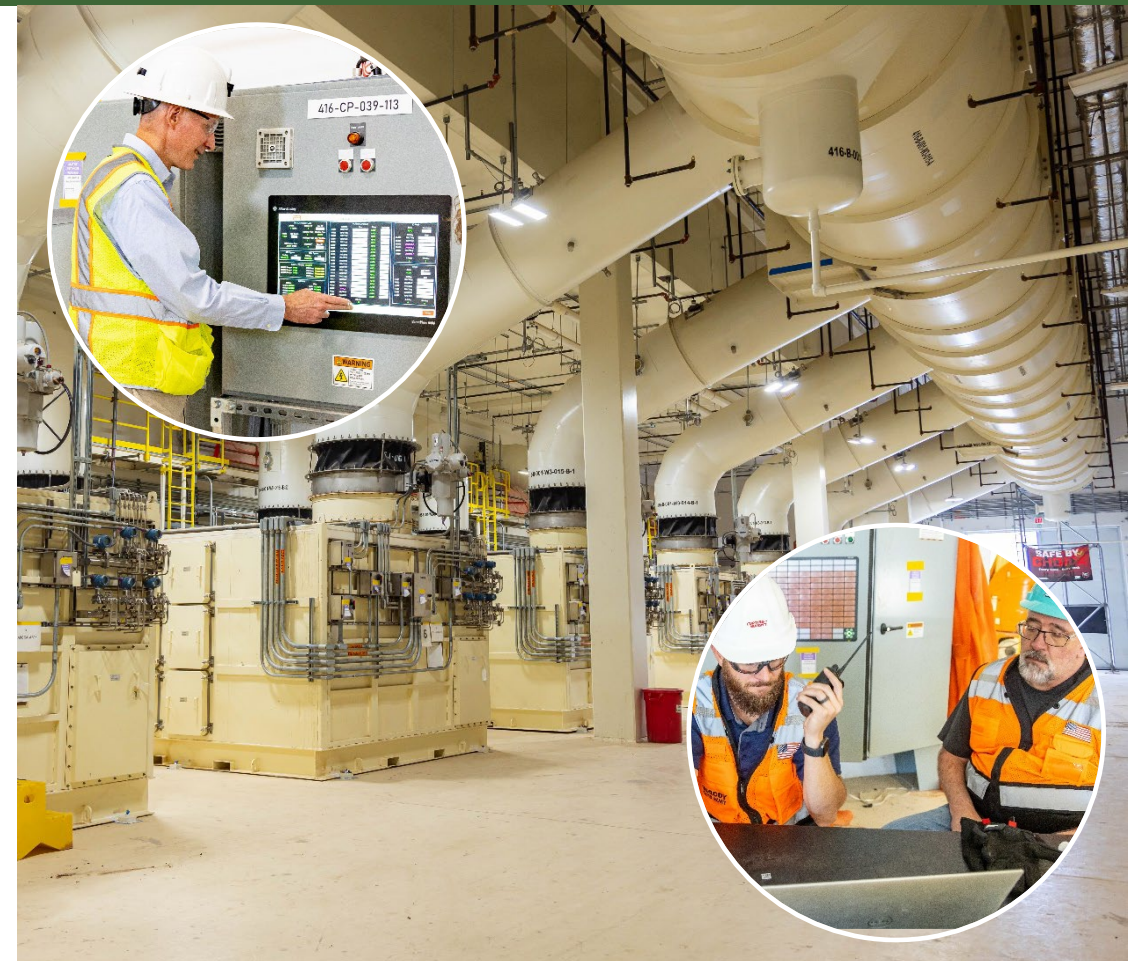
Above: Filter banks inside the SSCVS New Filter Building Inserts: Filter fan control panel (above), systems testing (below)
