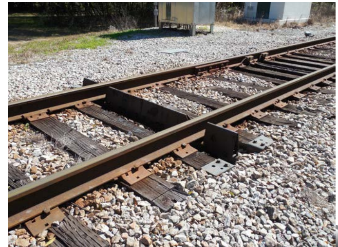
Dragging Equipment Detector
